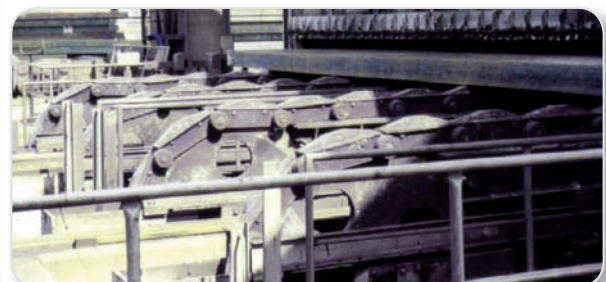
Special chain pitch 600 mm pre-heating brames. ( Oven temp. 500° C)
